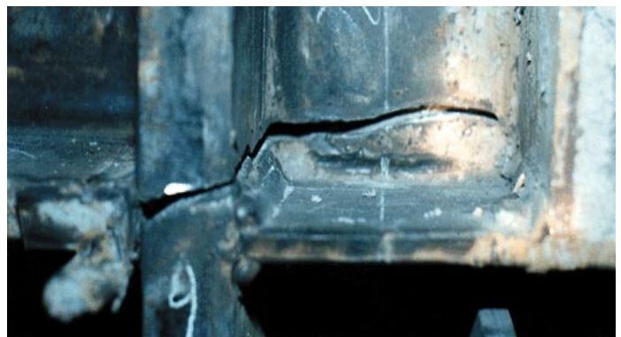
Typical connection fracture in a moment-frame building.
