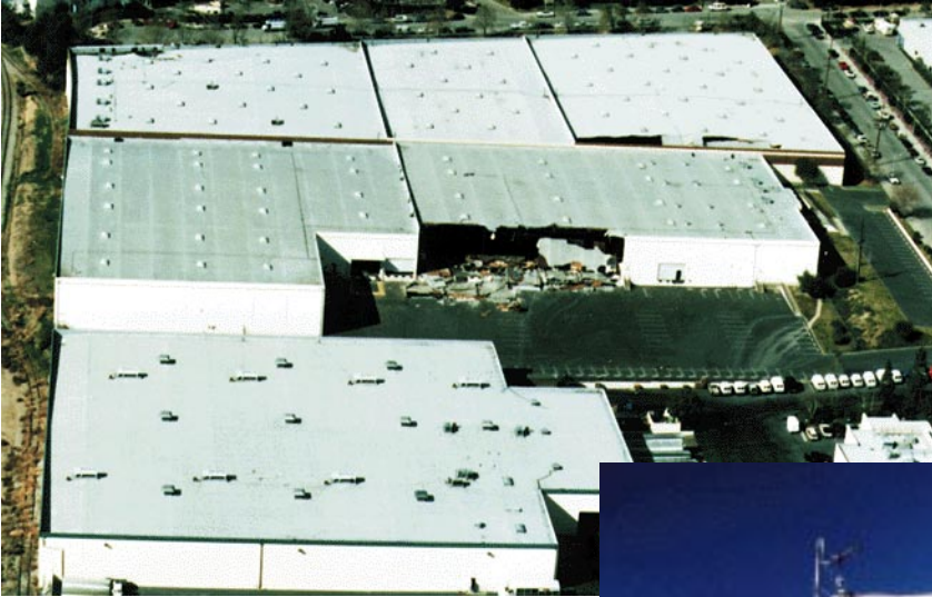
Typical tilt-up wall and roof failure due to out-of-plane loads.
